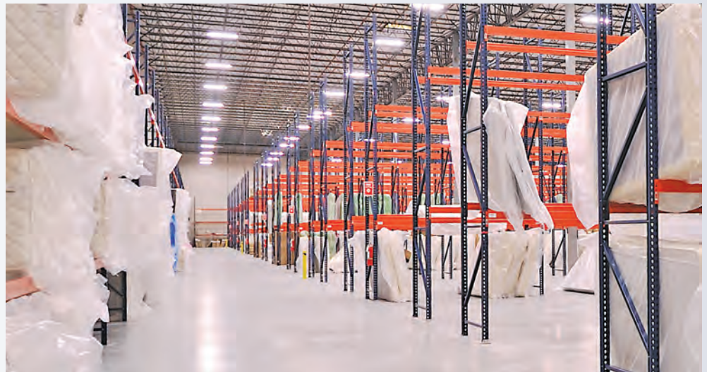
For Mattress Giant's 80,000 square foot facility in Davenport, FL, TriFactor provided and installed heavy-duty teardrop pallet racking with various load capacities to accommodate three-level storage.
