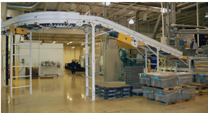
Horizontal powered conveyor taking discharged ingredient totes from a vertical lift conveyor and declining the totes to the respective mixer.
